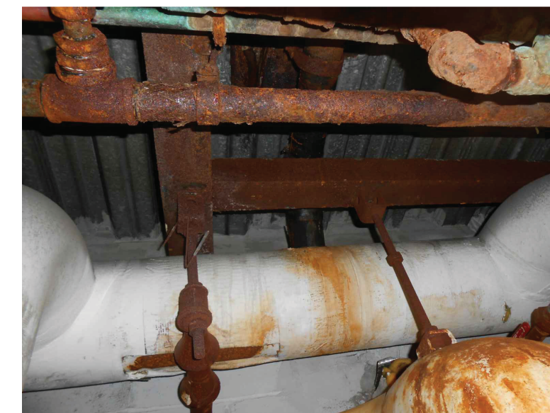
CORRODED PIPING AT MECH. RM.
