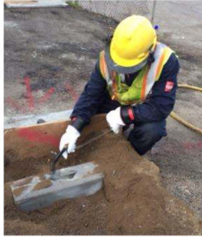
Break out window on each top duct found. Strike Away From the center.
