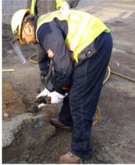
Find edges & visualize all ducts. Remember that There could be several across and underneath. Keep area clean, so you can tell configuration.
