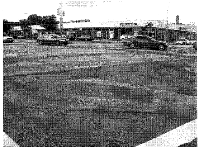
Photo No. 34 – View of Moderate Risk Site No. 32, Manhole #8134, Queens Boulevard and Hillside Avenue, Map ID 32.
