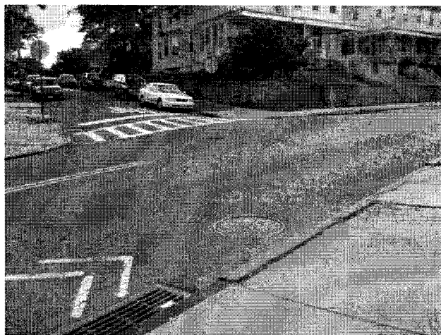
Photo No. 11 – View of Moderate Risk Site No. 9, Manhole 17206, Parsons Boulevard and 86th Avenue, Map ID 52.
