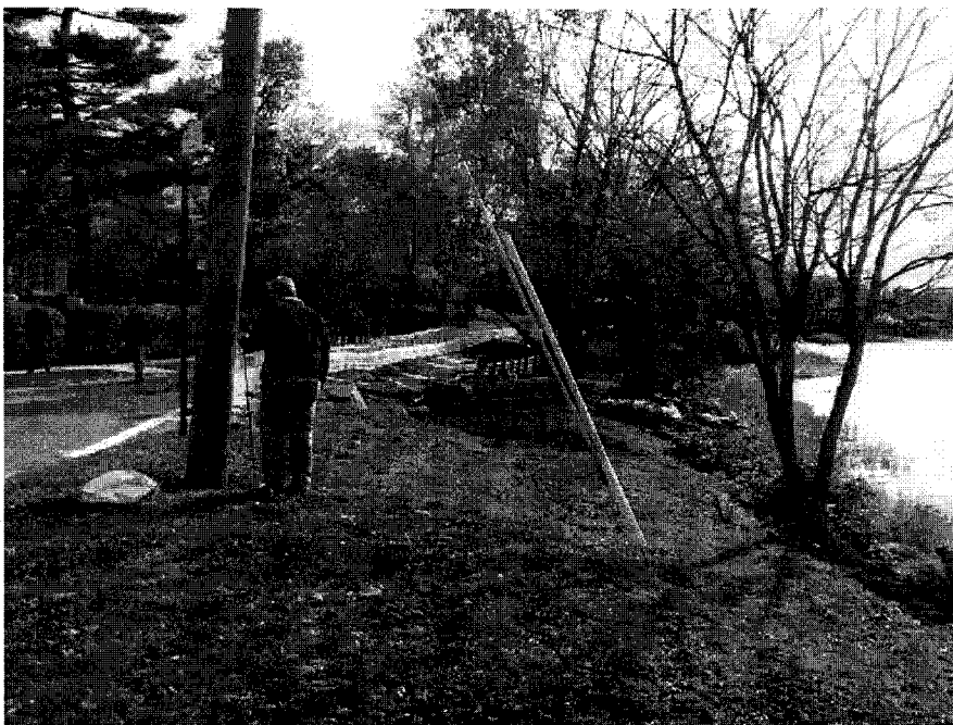
Photo 15. View south from the west side of the Shore/Manor road intersection showing the Outfall No. 6 location and Collapse No. 2.
