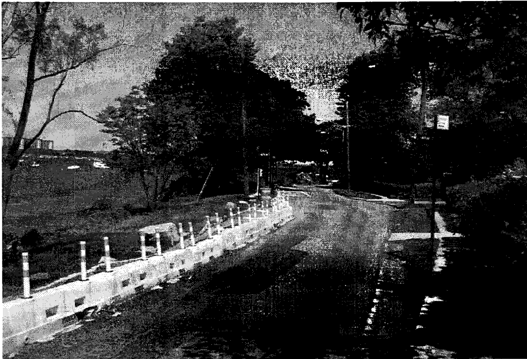
Photo 14. Looking north along Shore Road from midway between Manor Road and Hollywood Avenue. Collapse No. 2 is at the left (west). Outfall No. 6 location is at the foot of Manor Road, to the left (west) of the orange plastic pylon.
