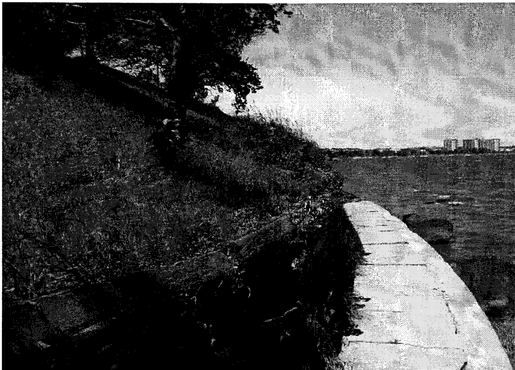
Photo 2. Looking west toward proposed Outfall No. 1 location, north of the foot of West Drive. Note timber retaining wall and concrete foundation.
